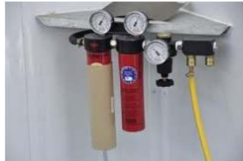
Figure 1. Compressor & Air Filter
