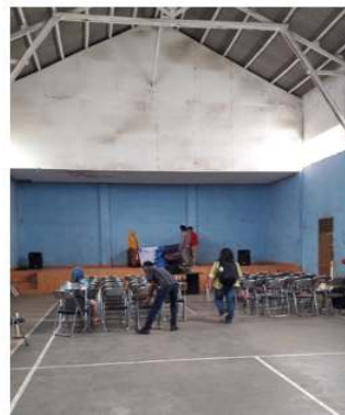
Figure 4. Community meeting place that needs renovation and structure strength investigation due to earthquake and landslide disaster occurrence
