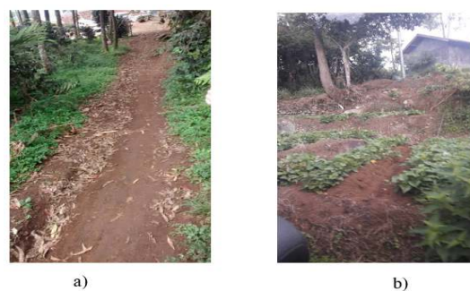
Figure 2. Condition of village road, soil road, steep and slippery during rainfall occurrence (a) and landslide prone retaining wall near housing area
