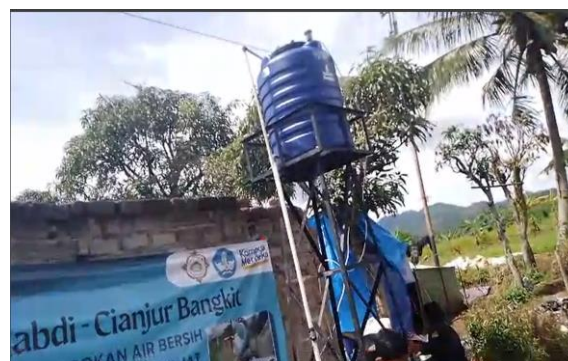
Figure 2 Facility drilled wells and water tower
