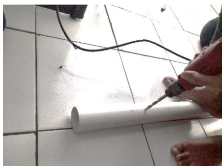
Figure 14. Perforation at the bottom of the pipe for water ventilation
