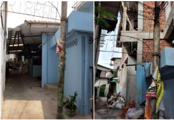
Picture 20. Before renovation of the northwest corner of Mushollah Al Ikhlas (left) and after renovation (right)
