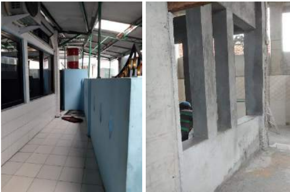
Picture 21. Before renovation of the east side of Mushollah Al Ikhlas (left) and after renovation of window openings (right)
