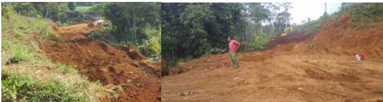
Picture 1. Road and slope conditions to be improved
