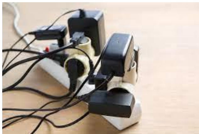
Figure 1. examples of incorrect use of electricity
